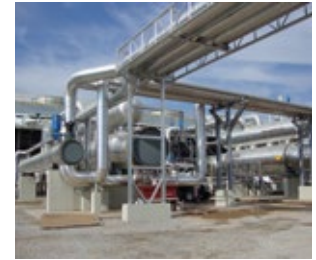
Turkey Geothermal power Dora II
